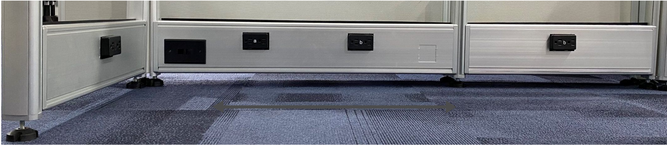
Typical Electrical Raceway (covered)
