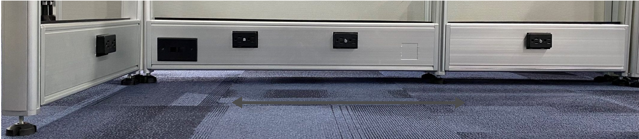
Typical Electrical Raceway (covered)
