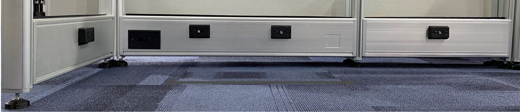
Typical Electrical Raceway (covered)
